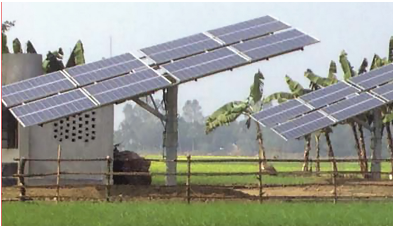
Double-axis tracking. Solar irrigation pump systems using manual double-axis tracking standers (photo provided by Asian Development Bank consultant).
