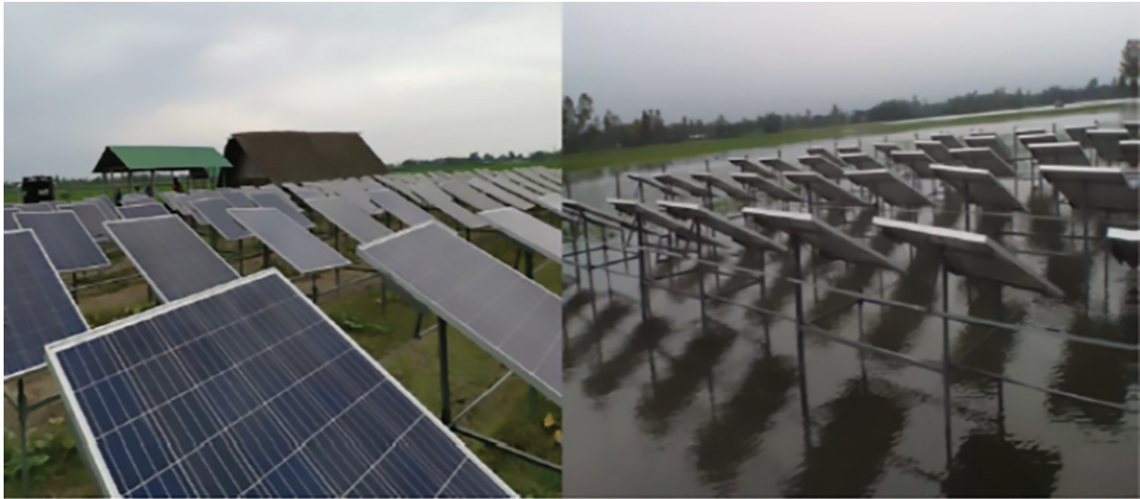
Single-axis tracking. Solar irrigation pump systems using manual single-axis tracking standers (photos provided by Asian Development Bank consultant).
